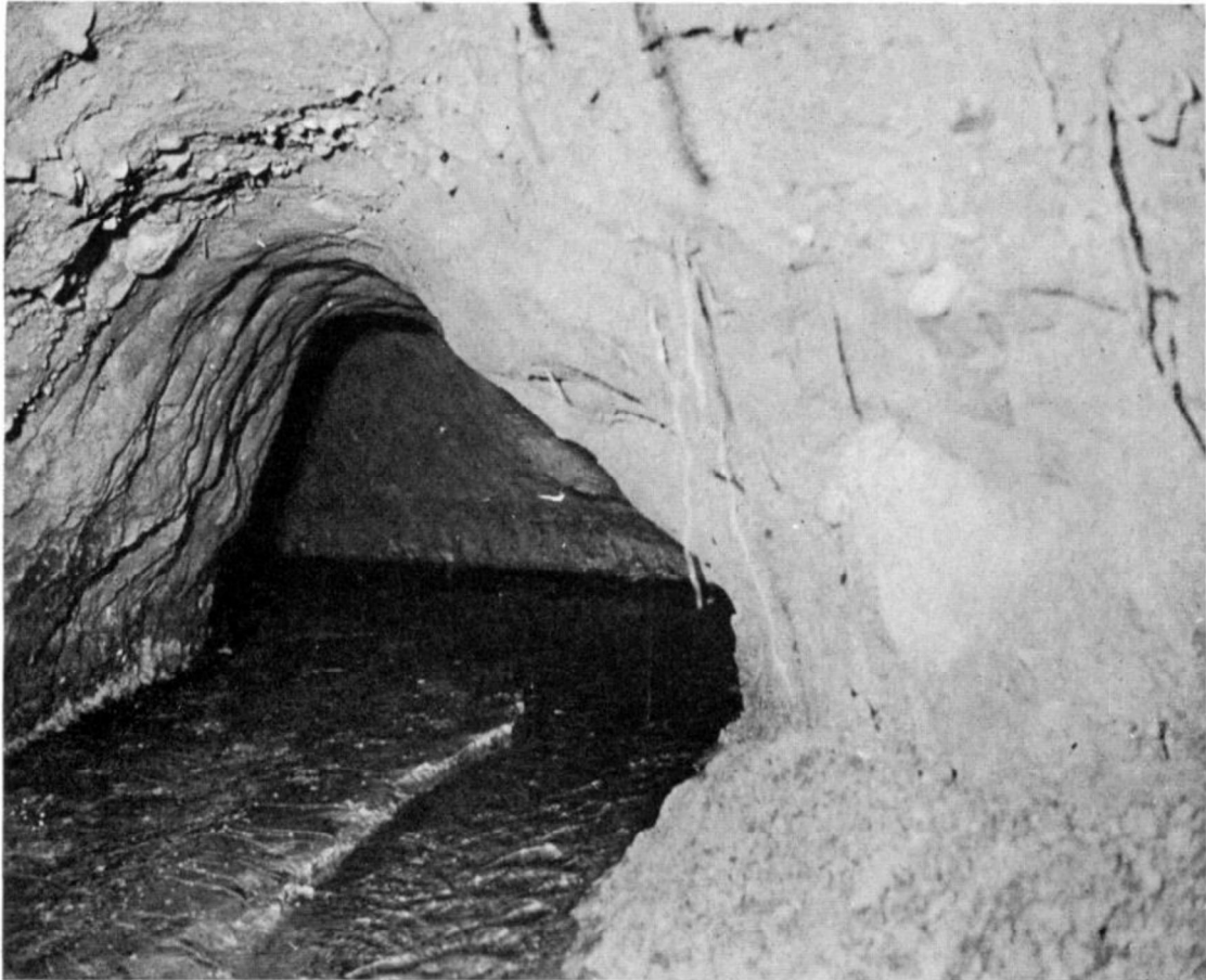
Fig. 3. Water emerging from underground tunnels.
